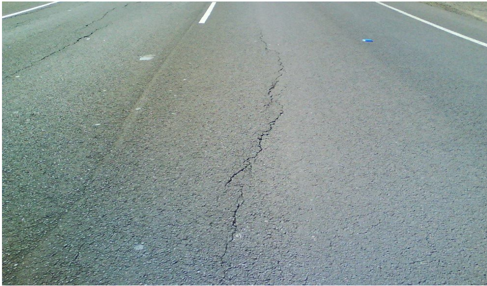
Figure c.4 Longitudinal distress in asphalt Pavement
