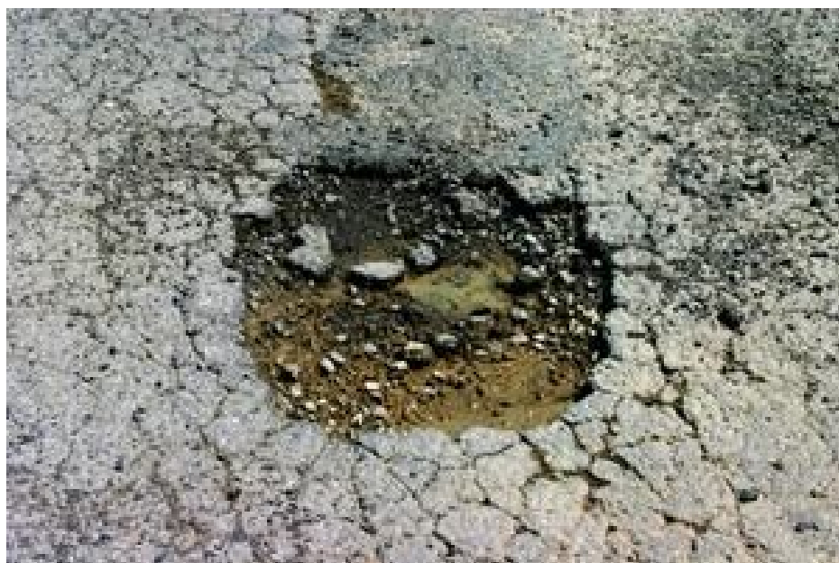
Figure c.5 Pothole distress in asphalt Pavement
