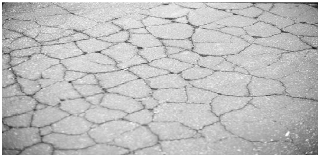
Figure c.1 Fatigue (alligator) cracking in asphalt pavement
