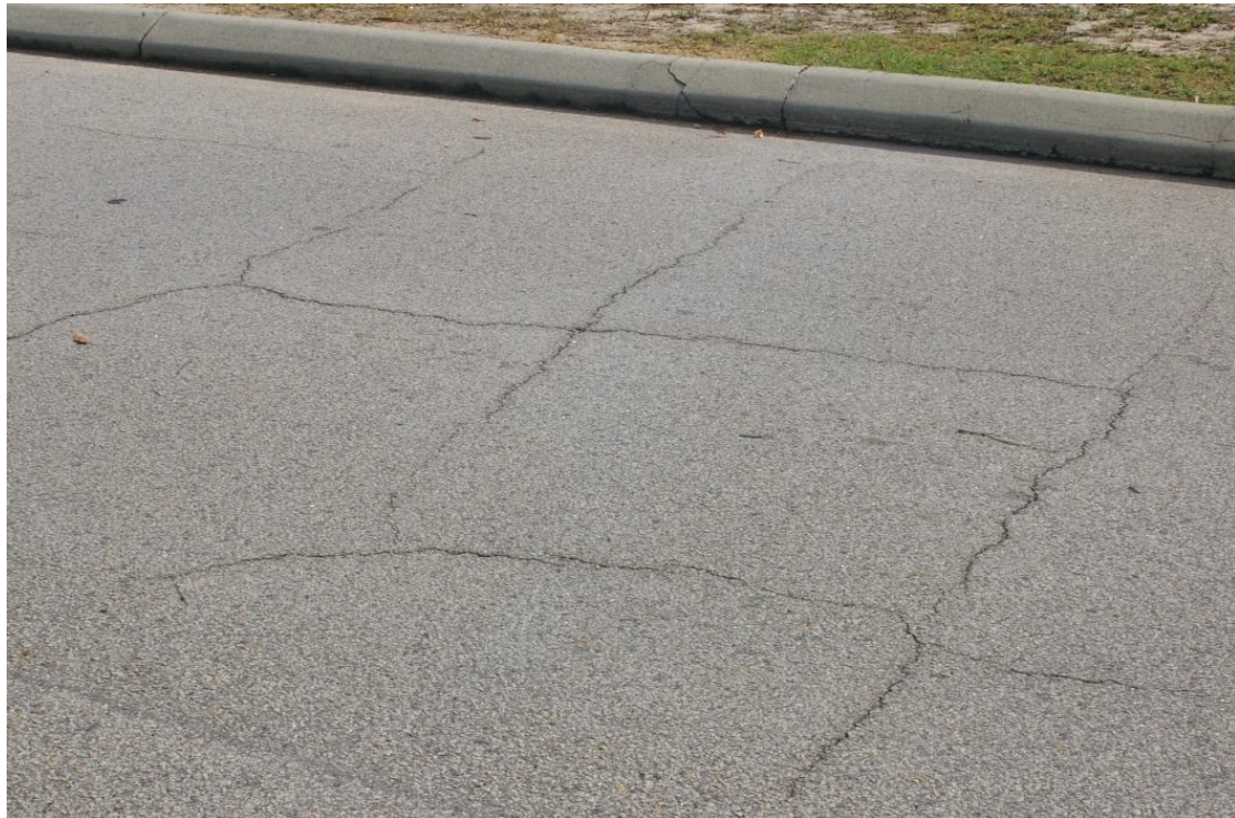
Figure c.3 Block distress in asphalt pavement
