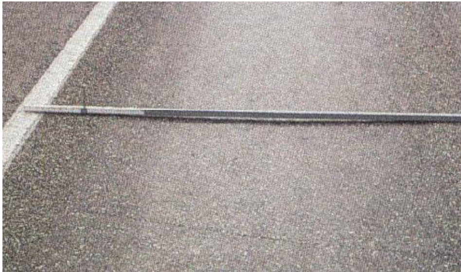
Figure c.6 Rutting distress in asphalt Pavement
