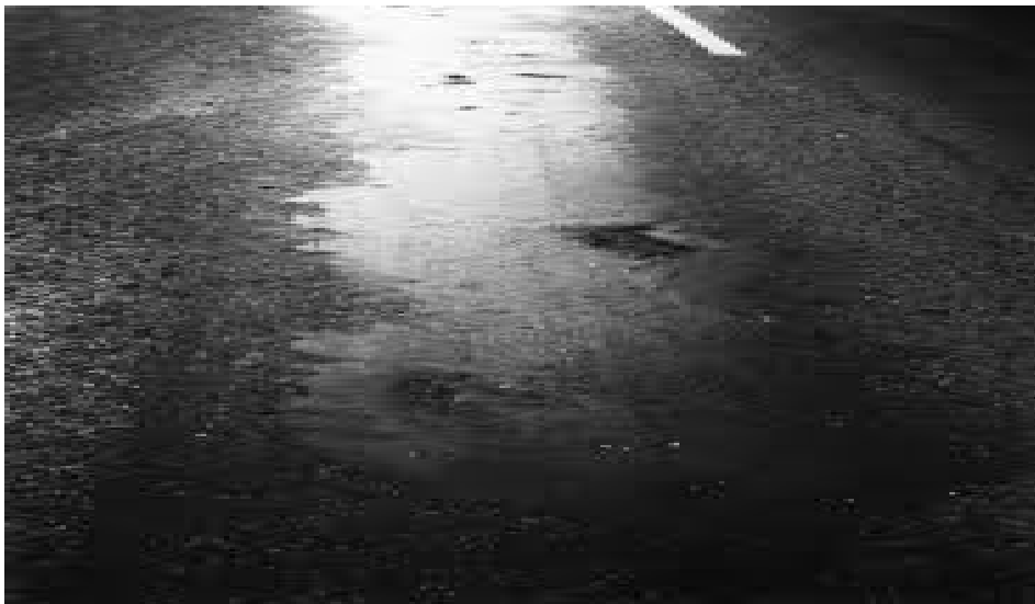
Figure c.2 Bleeding distress in asphalt pavement
